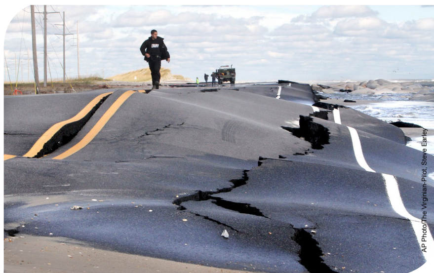
Storm surge on top of rising sea levels have damaged roads and other coastal infrastructure.
