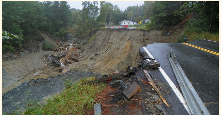
Figure 5.6. Vermont Route 131, outside Cavendish, a week after Tropical Storm Irene unleashed severe precipitation and flooding that damaged many Vermont roads, bridges, and rail lines. (Photo credit: Vermont Agency of Transportation).
